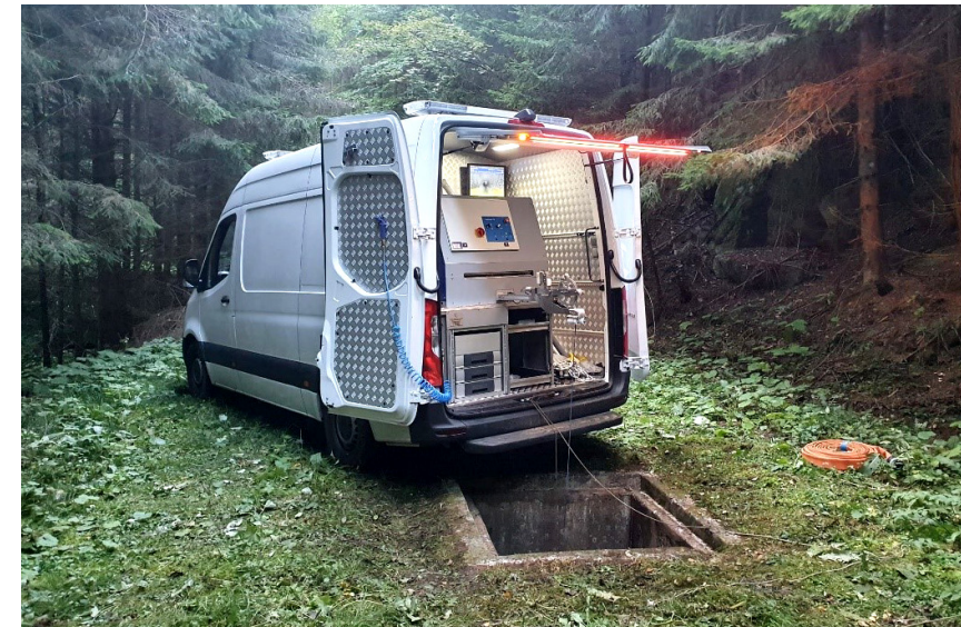
power plant pipe, access in a forest
